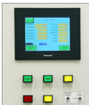
User interface – failure position light panel and count screen
